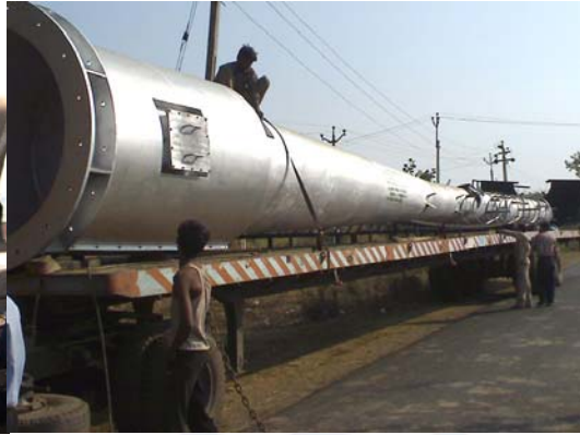
Self Supported Chimney
