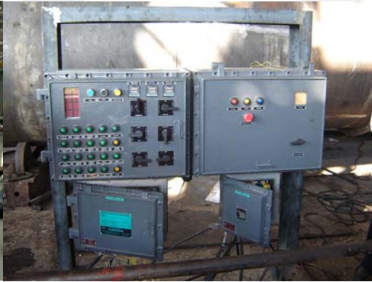
Explosion Proof Control Panel
