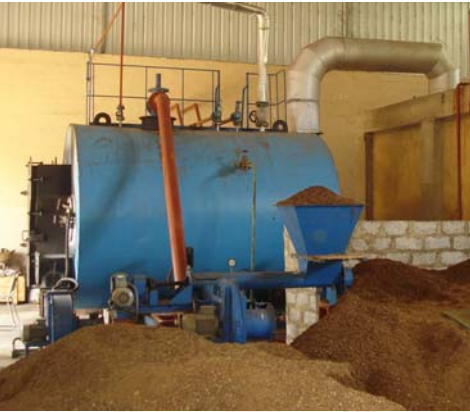
Husk Fired Boiler
