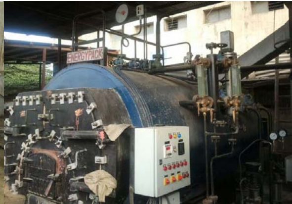
Brette Firing Boiler
