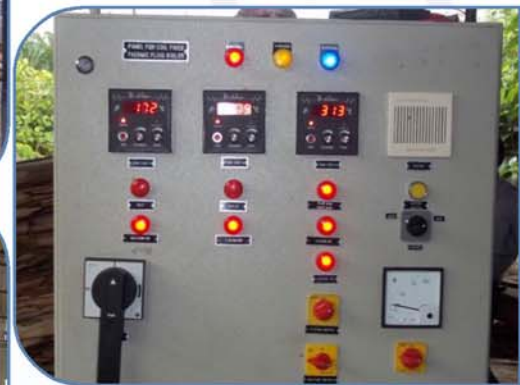
Control Panel For Automatic Operation
