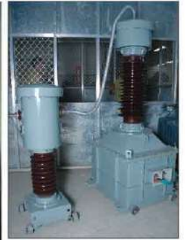
High Voltage Testing
